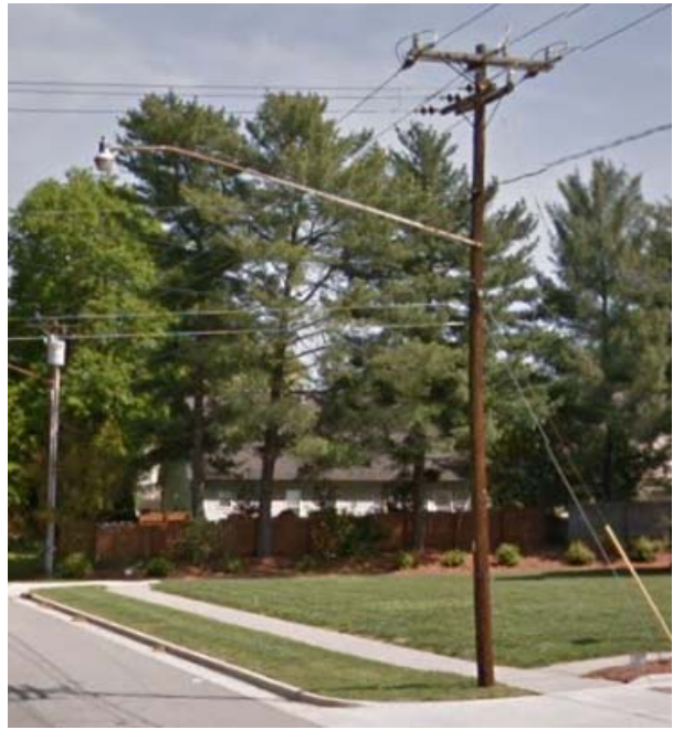
STREET LIGHT ON EBERT STREET
