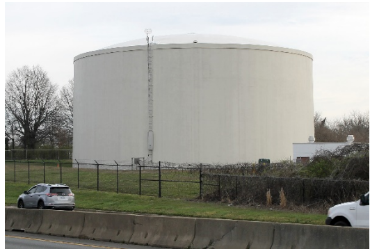
US 52/Liberty Street Water Tank
