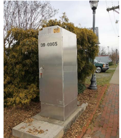
Traffic Signal Box
