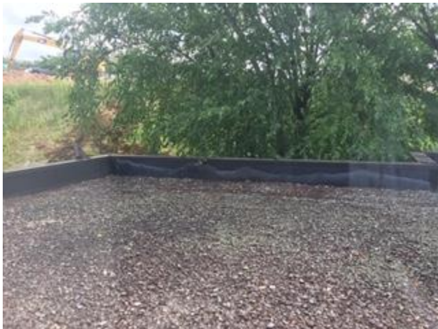
EDPM pulling away from parapet wall in multiple locations throughout roof
