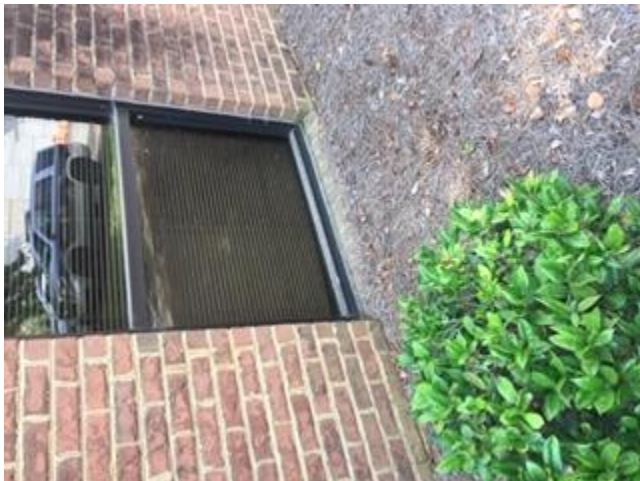
Base of windows need to be excavated to alleviate potential flooding
