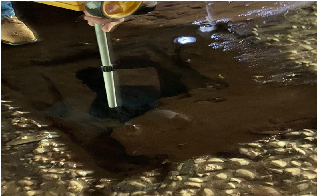
Remains of wooden piers in the floor of the culvert
