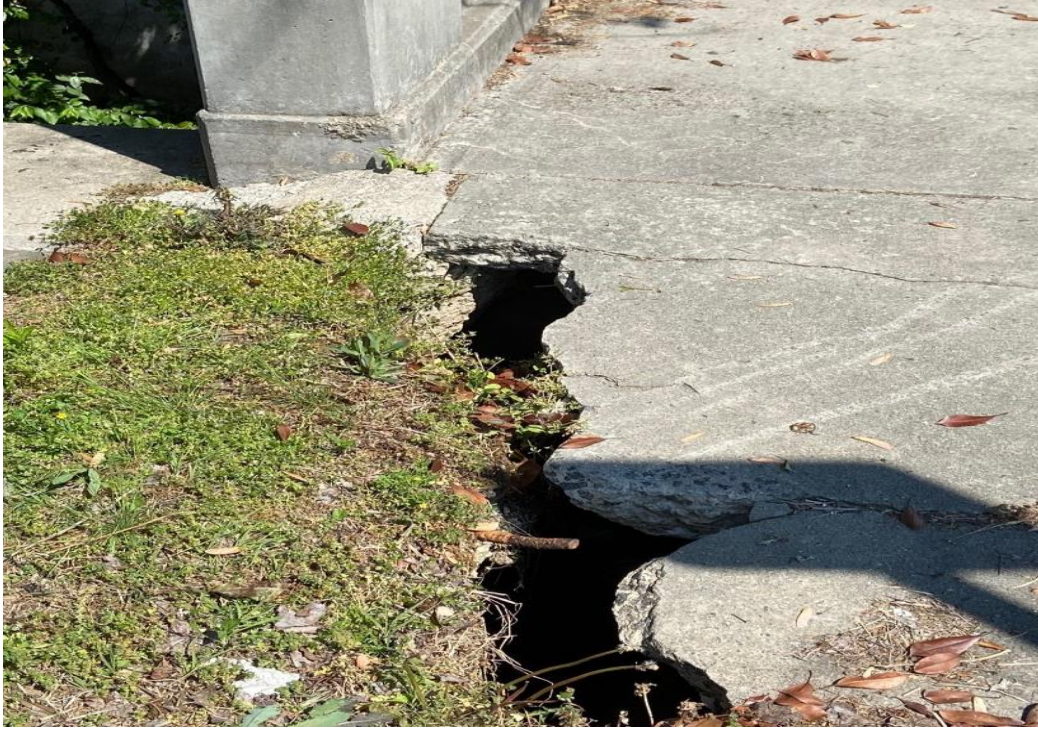
Sinkhole at the sidewalk
