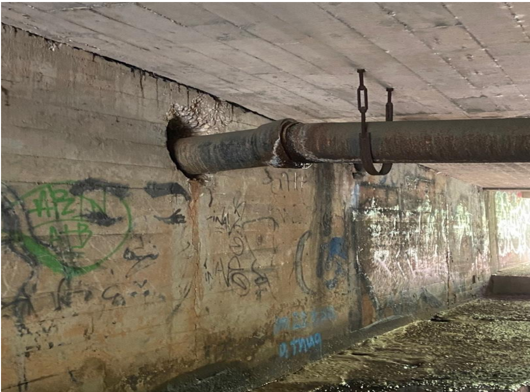
Damaged waterline from failing culvert wall
