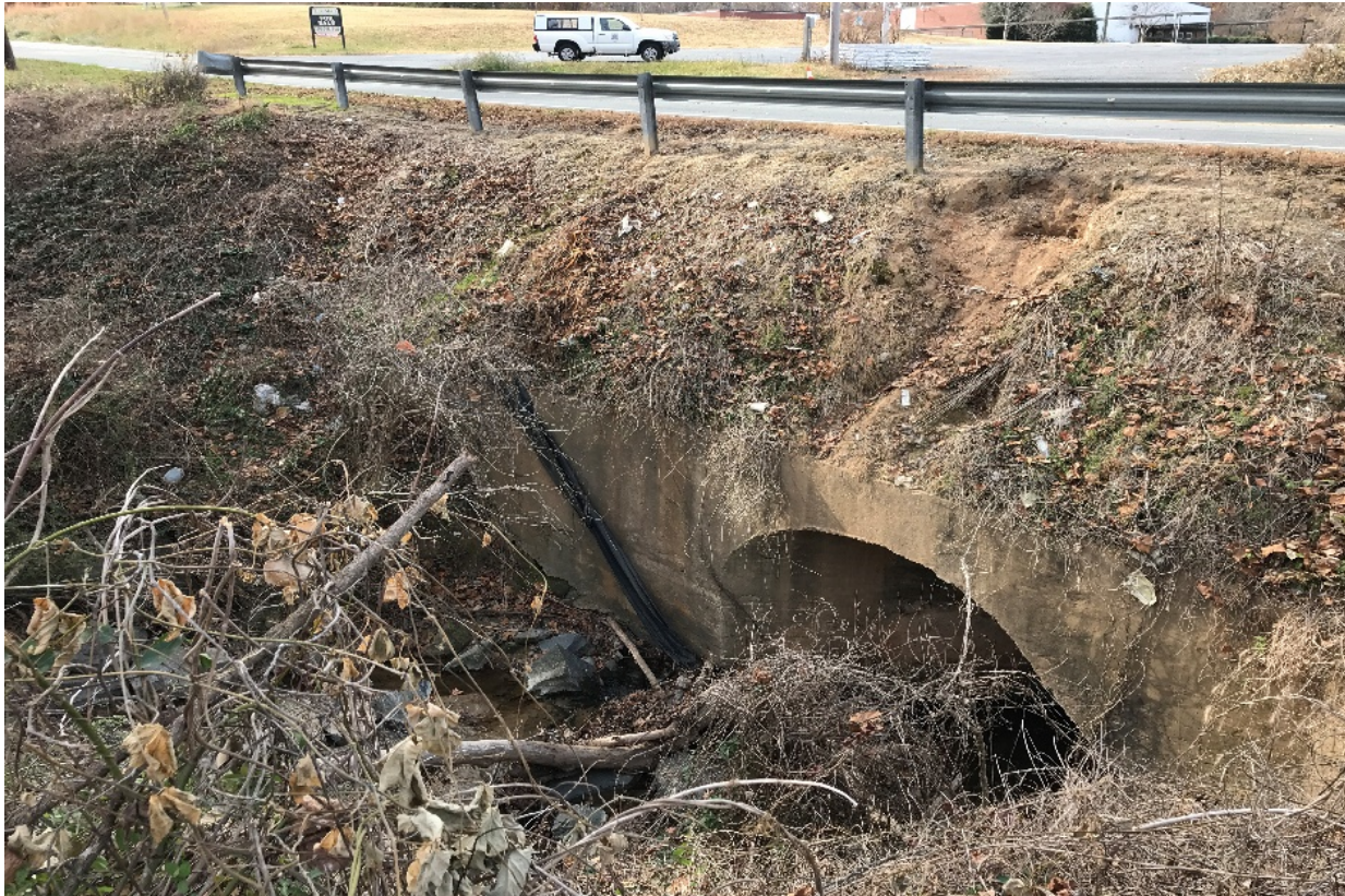
Eroding slopes over box culvert – Work Area B
