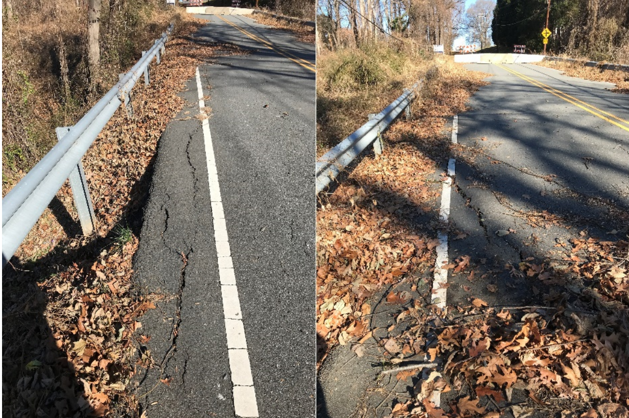
Longitudinal cracking and undermined guard rail along edge - Work Area A
