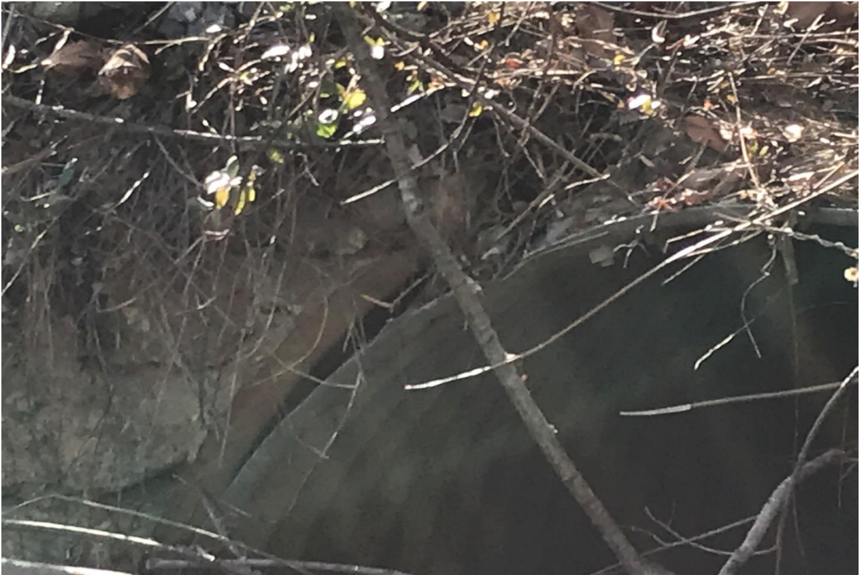
Pipe pulling away from the surrounding soil.
