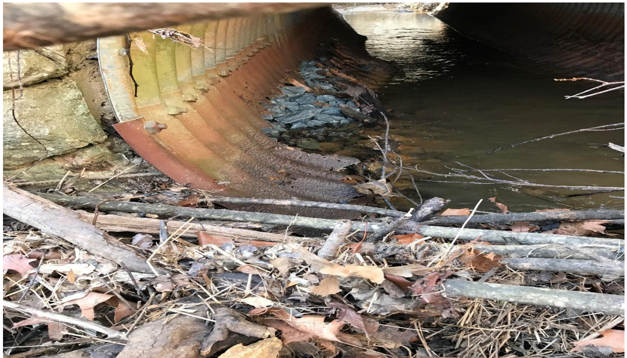
Upstream side of culvert (note: invert of culvert is gone)
