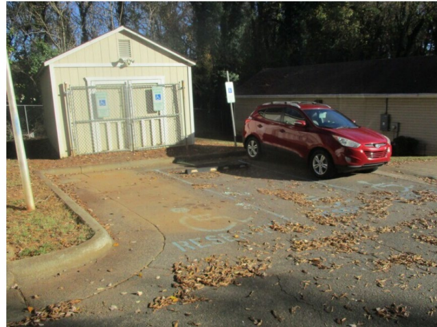
1. (7.1-01) Designated van-accessible parking space not present. No access aisle present. Van-accessible placard not present at the parking area serving the leasing office. (ADA)
